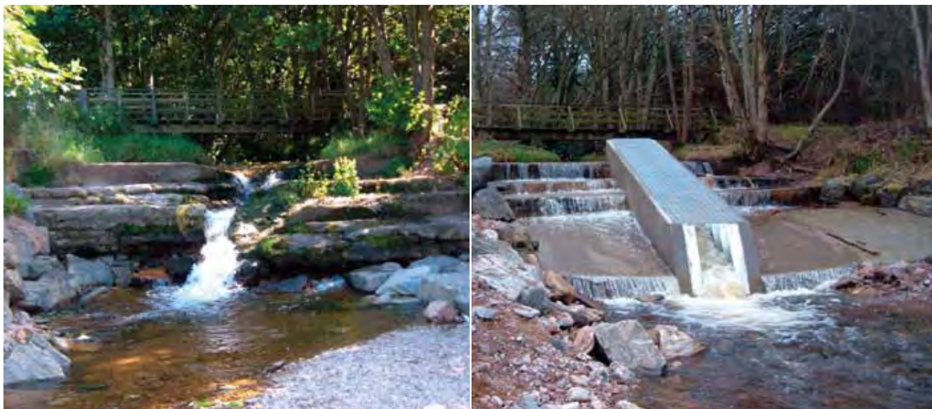
Before (left) and after shots showing improvements to a fish pass on the Spey River, one of the CASS project’s actions that has opened up 150 km of salmon habitat in Scotland
