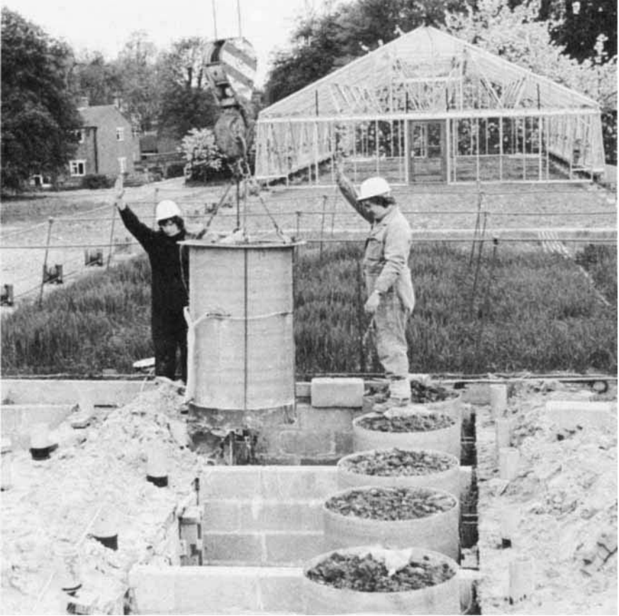
PLATE 3. Installation of a complete lysimeter. The permanent steel base, with a drainage outlet and the hooks for lifting, can be seen. The pipes at 50 cm depth are connected to supplementary drainage outlets in the clay monoliths (see text).
