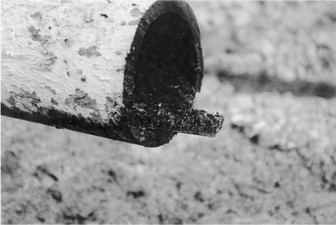
Fig. 15. Solid clog material buildup inside temporary toe header.
