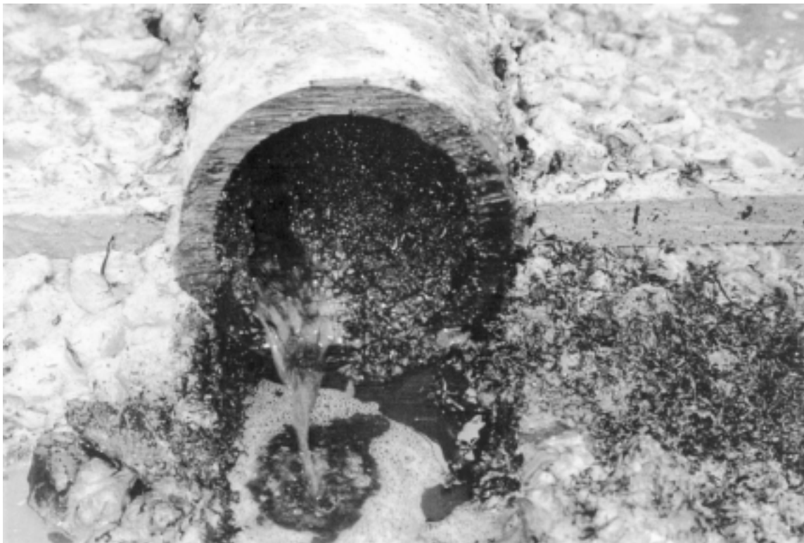
Fig. 13. Clog material inside temporary toe header (1994).
